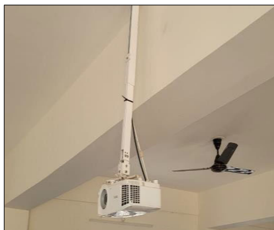
Figure 17: Showing projector installed in the class
